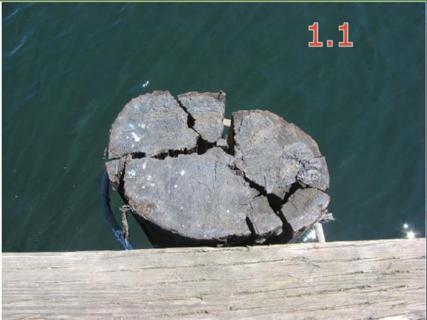
DESCRIPTION OF PILE: Decayed and split at top LOCATION: Typical multiple locations
