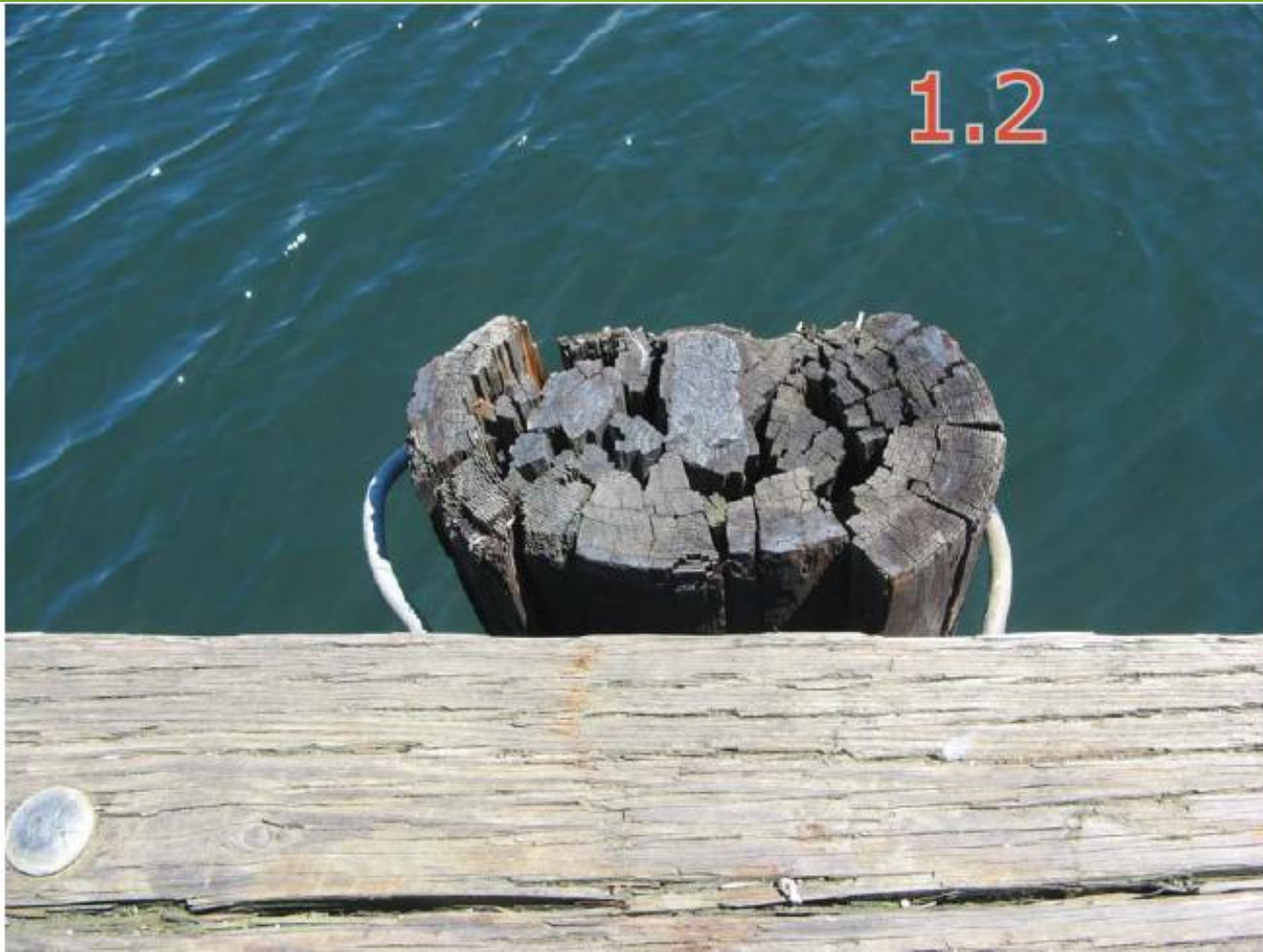
DESCRIPTION OF PILE: Crushed and decayed at top LOCATION: Typical multiple locations
